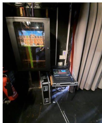
Stage left new equipment rack for AV and local audio control in the Great Hall
