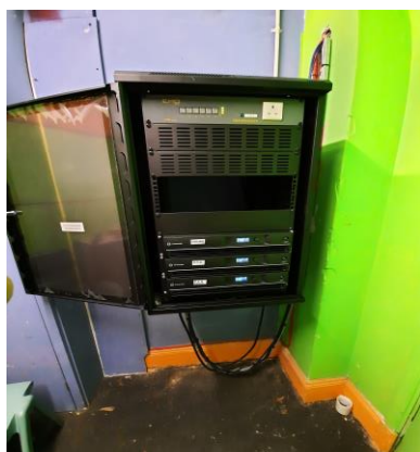
New DSP amplifiers for the Great Hall sound system now located in the green room.
